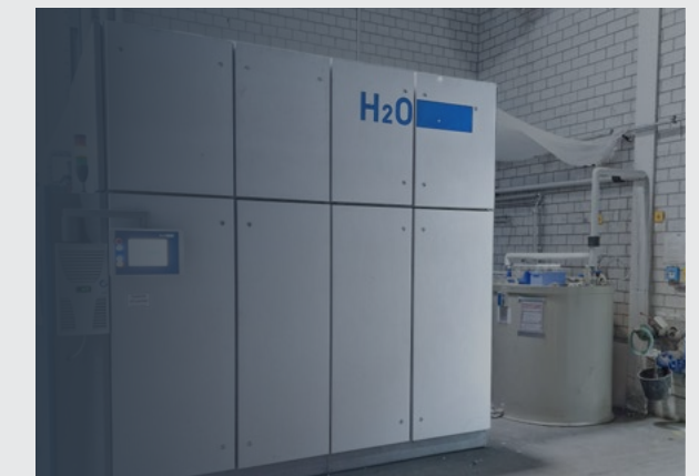
Evaporation plant at the Munich site
